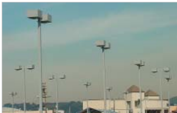
Low mounting heights often result in visual clutter as well as increased energy use.
